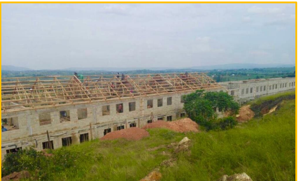
By June 7: Rafters extend halfway down the length of 100m long classroom bldg
