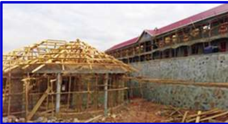
July 11: The Classroom Block ( upper rt. ) sports its new red roof. In front of the 2-level stone retaining wall is the portico being added to the front of the Administration Building.
