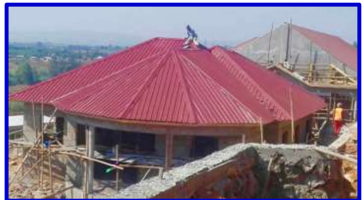
August 2: The Administration Building, which had rafters on July 11, now has its own new red roof. The dining hall is seen behind and to the right. View is from the Classroom Block.
