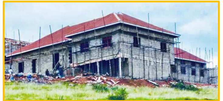
Below: May 31 st , the walls of the second floor of the classroom block are nearly built, and the roof of the dining hall is now complete.
